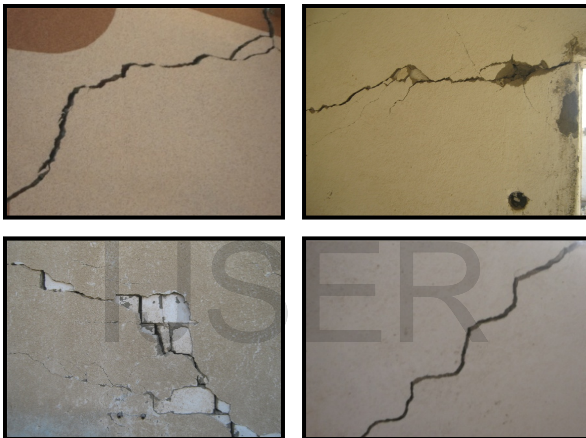
Fig. 2. Examples of structure damage caused by expansive soil in the study area
